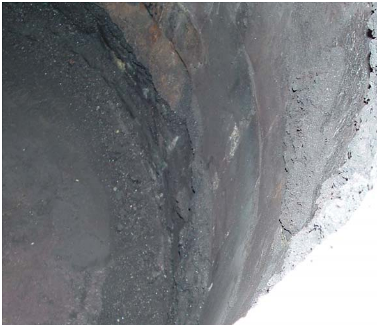
Figure 8: Viewed from the top it is clear that no significant wear of the lining has occurred.
